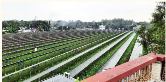
Visit to 3 MW solar power plant at Jamalpur
