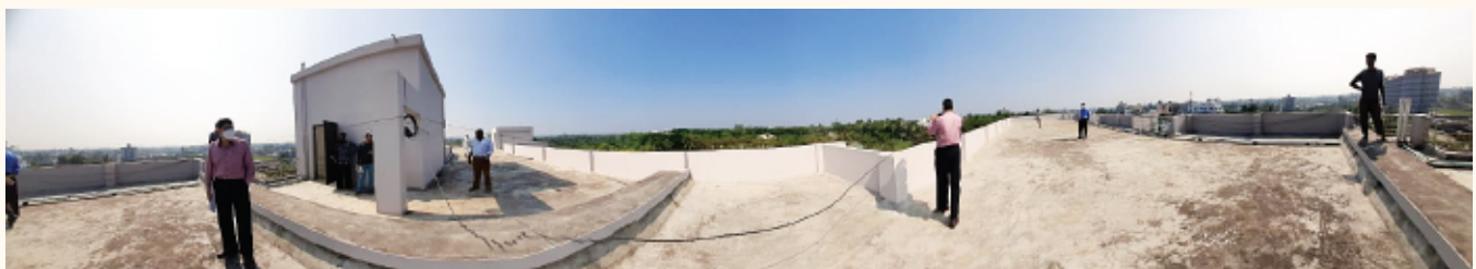
REEEP II team is inspecting the roof of Guest House of KU
