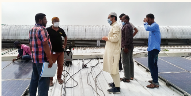
Visit to 300 kW Capacity Net Metered Rooftop Solar at the roof of DPQSL, Mymensingh
